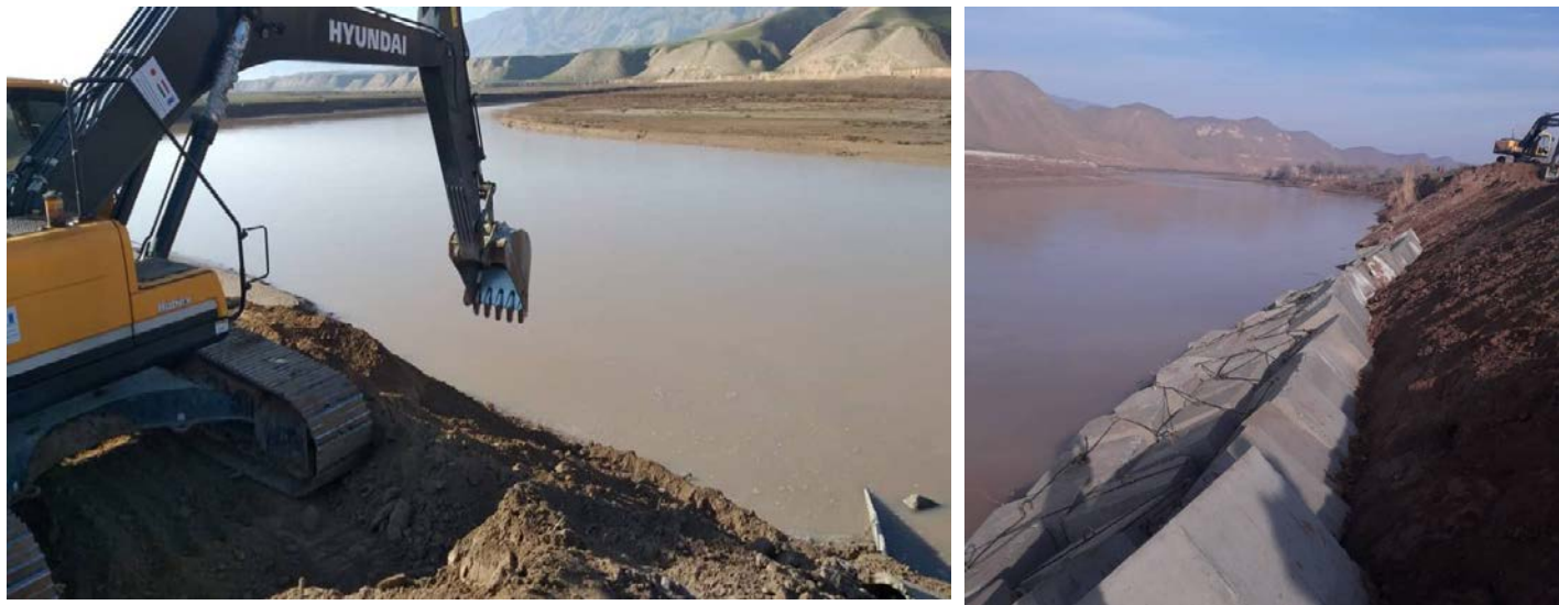
Figure 3-4. Implementation of pilot projects with the heavy machinery procured by the project
